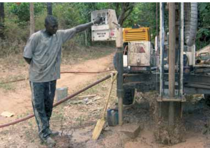
Borehole in Africa (Photo: Erich Baumann)
